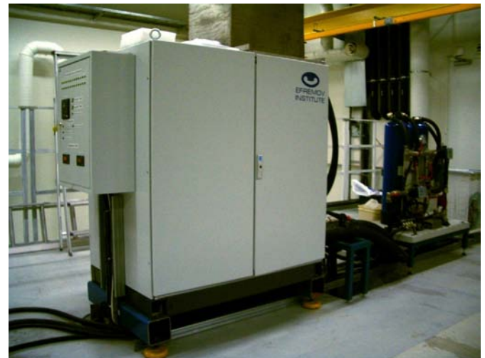
The water cooling and ion-exchange purification systems of the MCC-30/15 cyclotron
