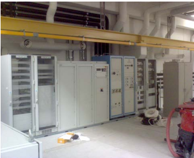
The supply and control systems
